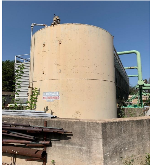
Photo Description: 10,000 gallon AST.
